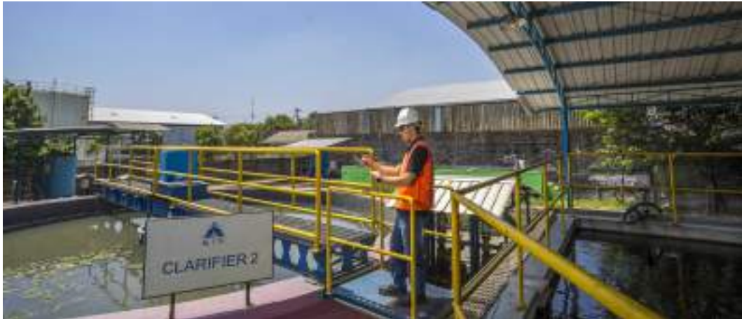
Gambar 9 Waste Water Treatment Plant
